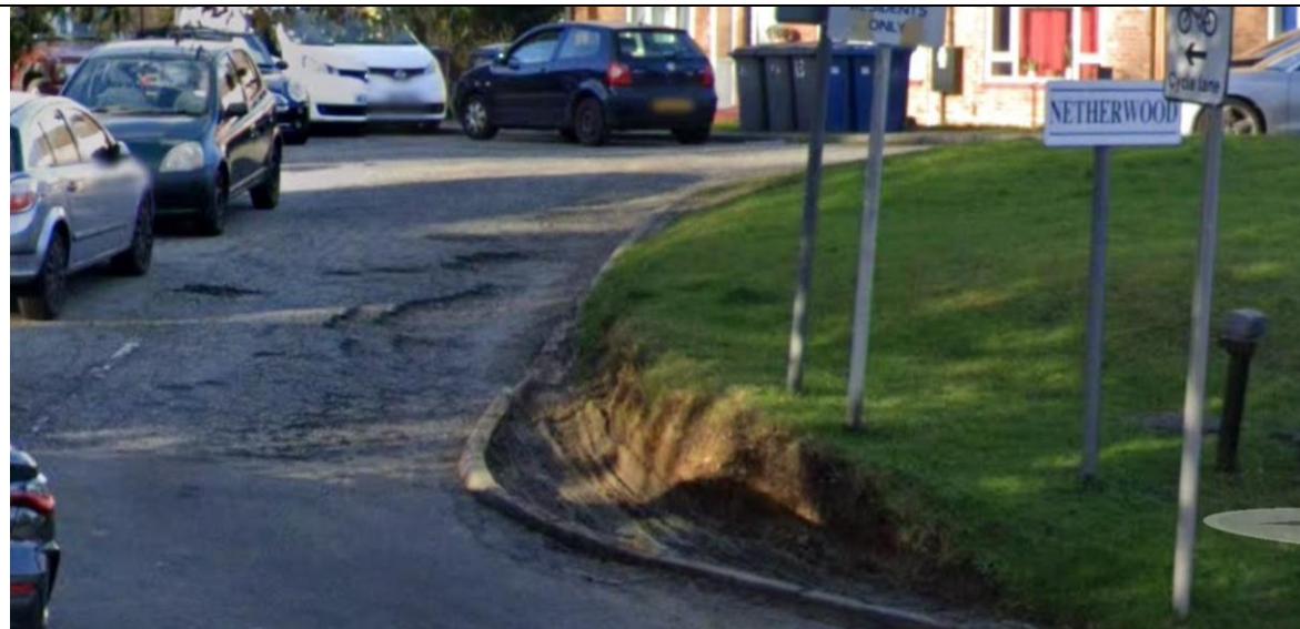
Figure 1 The potholes and state of the road, as well as damage to the side caused by refuse vehicles.
